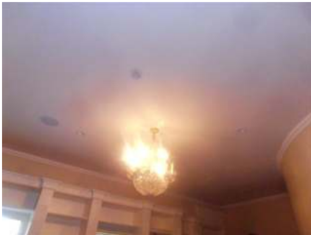
The ceiling lights in the office that are not working needs to be repaired.
